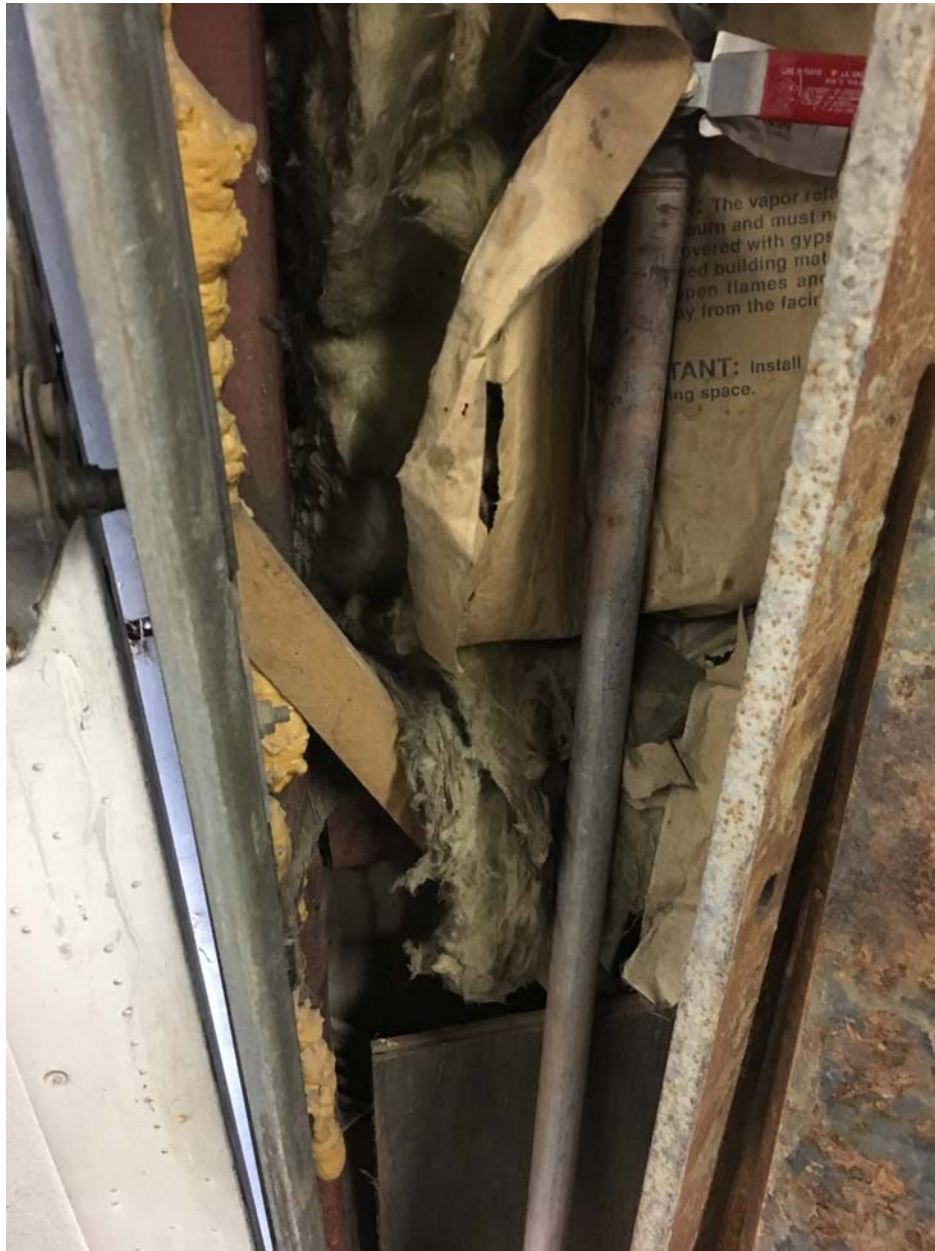
Photo #2 – Typical Damaged Insulation
