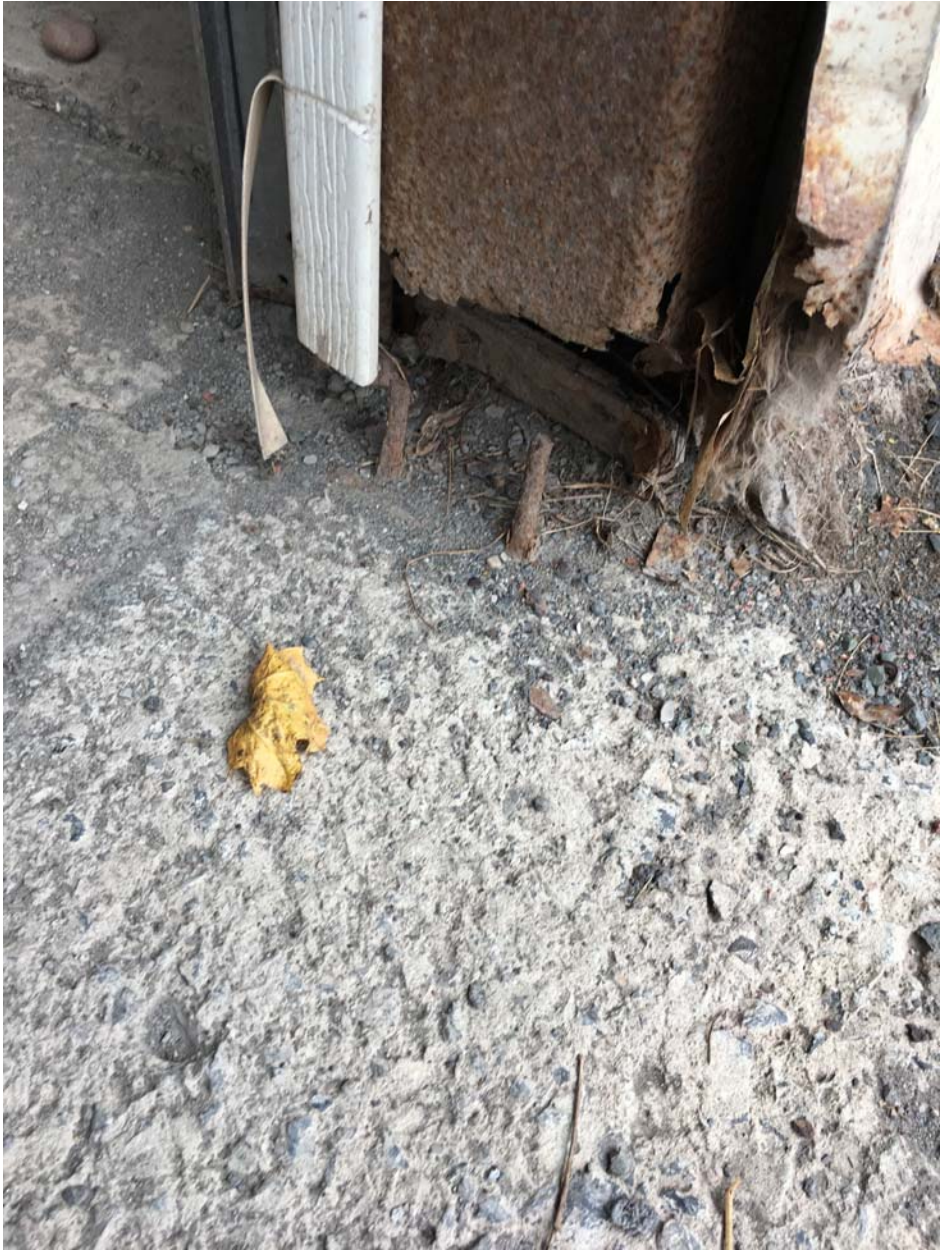
Photo #2 – Typical Example of Rusted Baseplate
